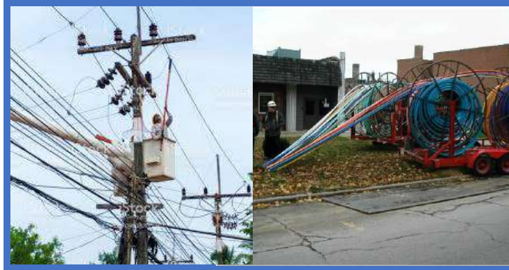
Electricity & IT infrastructure
